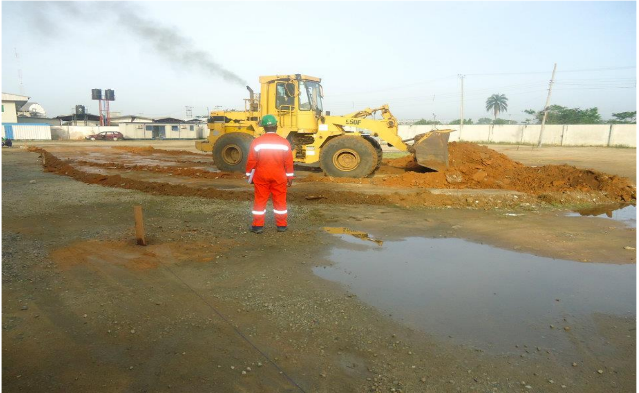
scrapping top soil in progress preparing to landscape (concrete flooring) Mykon ware house Trans-Amadi R.State
